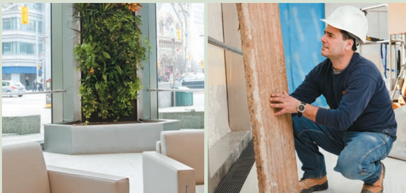
A section of one of the four “Living Walls.” Travertine from the original lobby floor being reclaimed for reuse.
